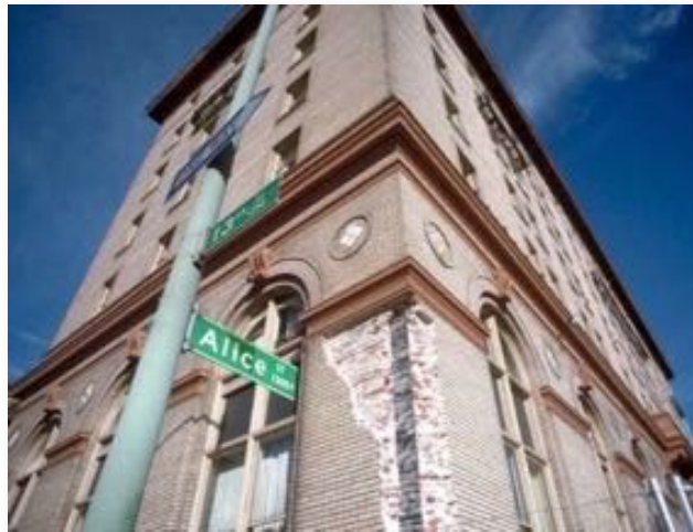
Cladding and Partition Failures
